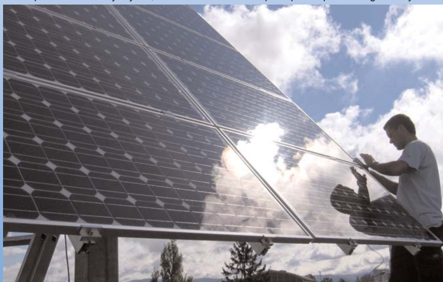
PV power plant on school roof
